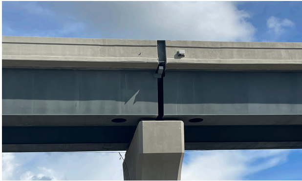
Ramp Bridge Barrier Electrical Junction Box, I-10 Loyola Interchange
